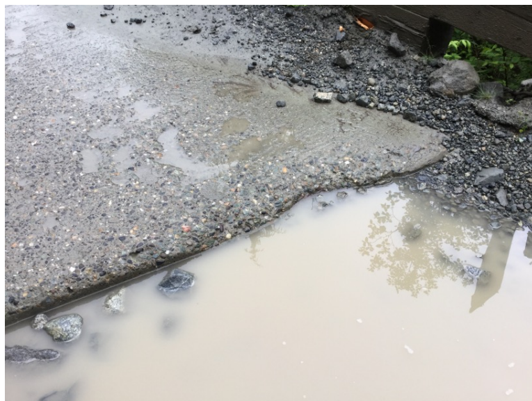
Concrete wear at downstream right bank
